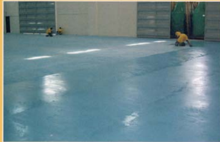
anti slip epoxy flooring
